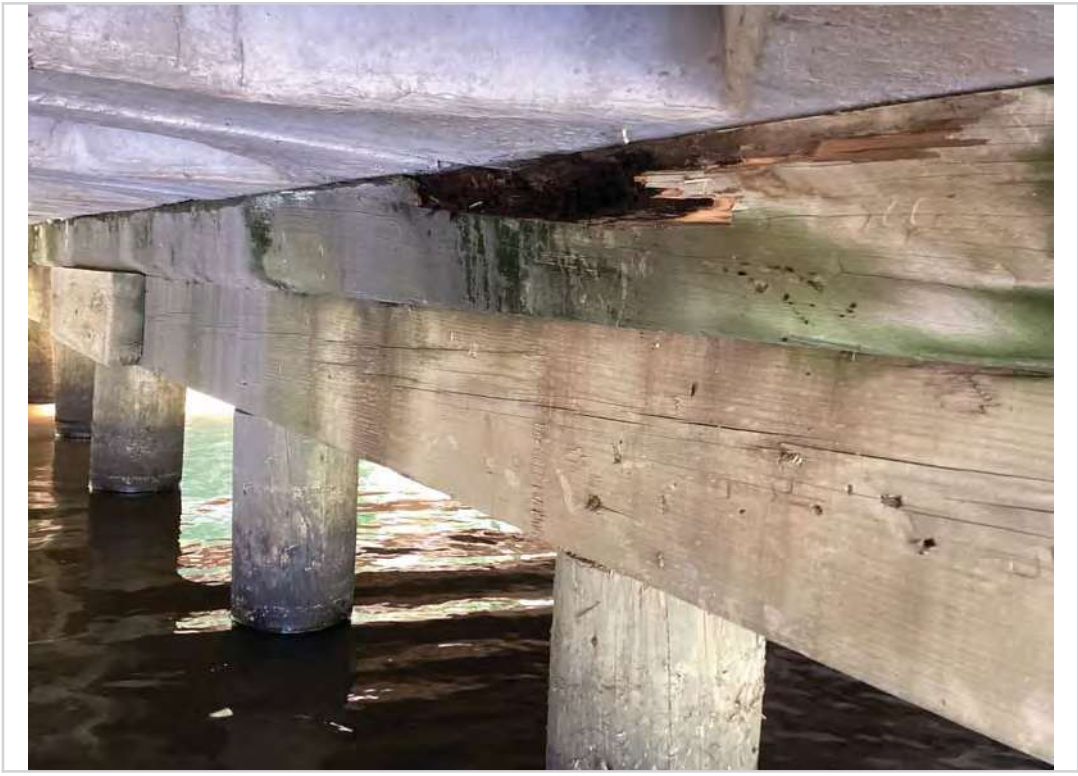
Bent 2 cap A decay
