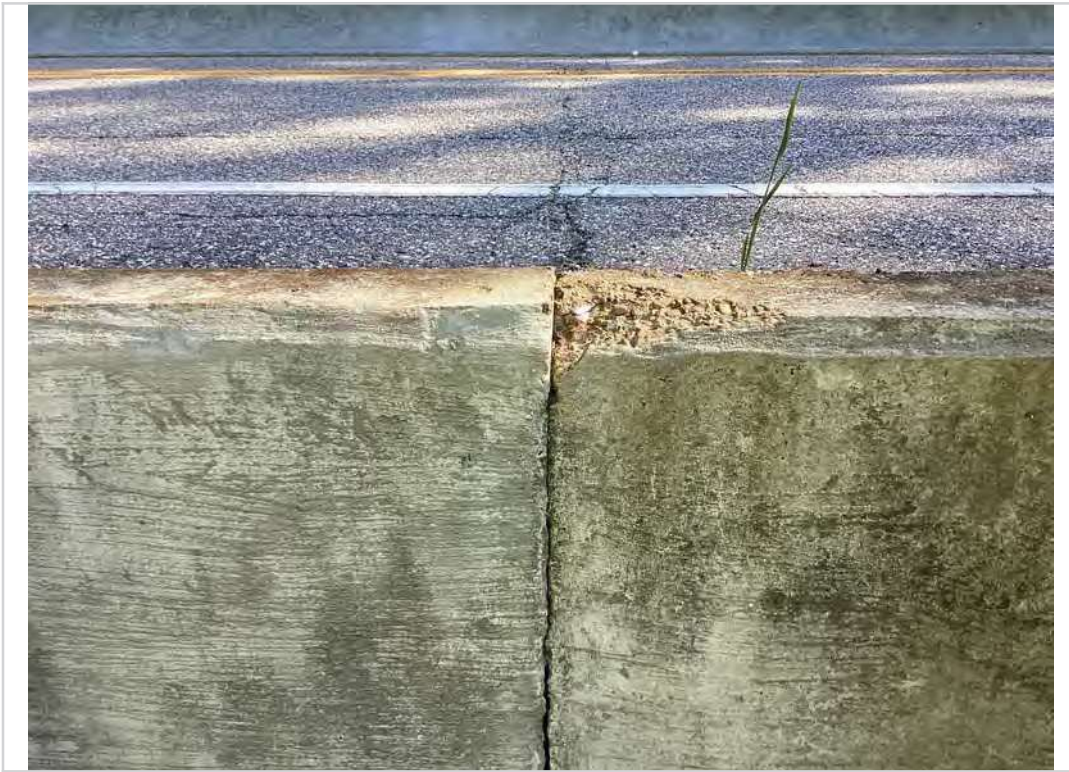
Span 1 left curb spalling
