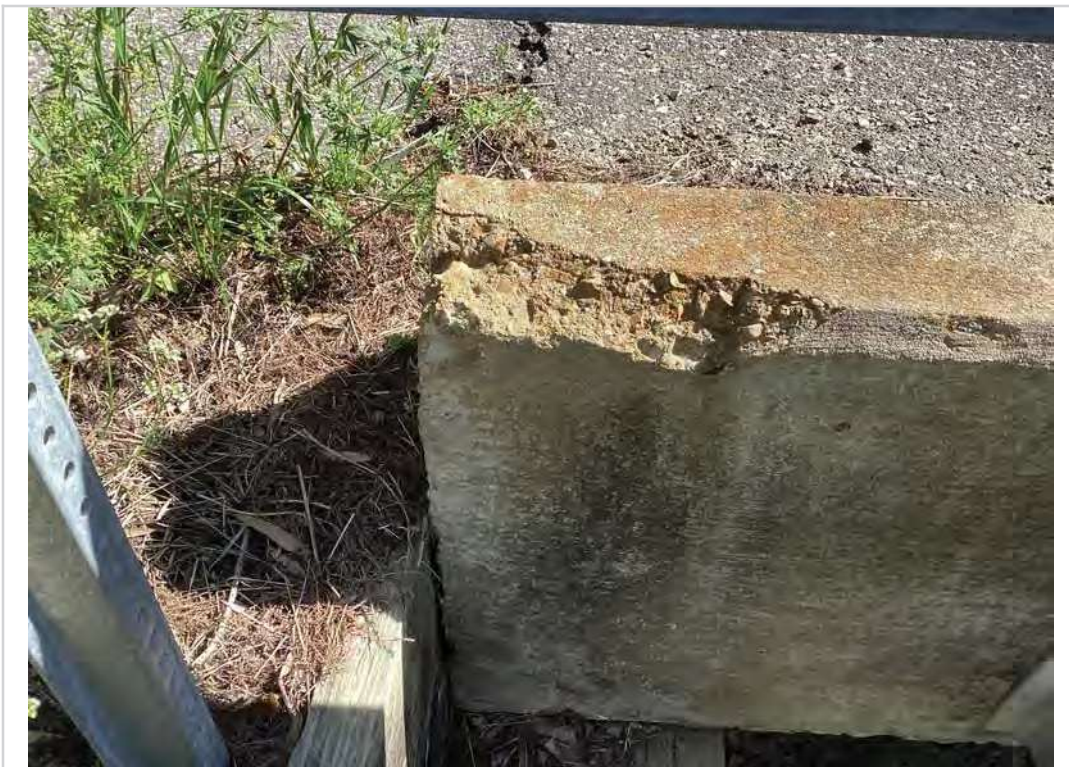
Span 2 left curb spalling
