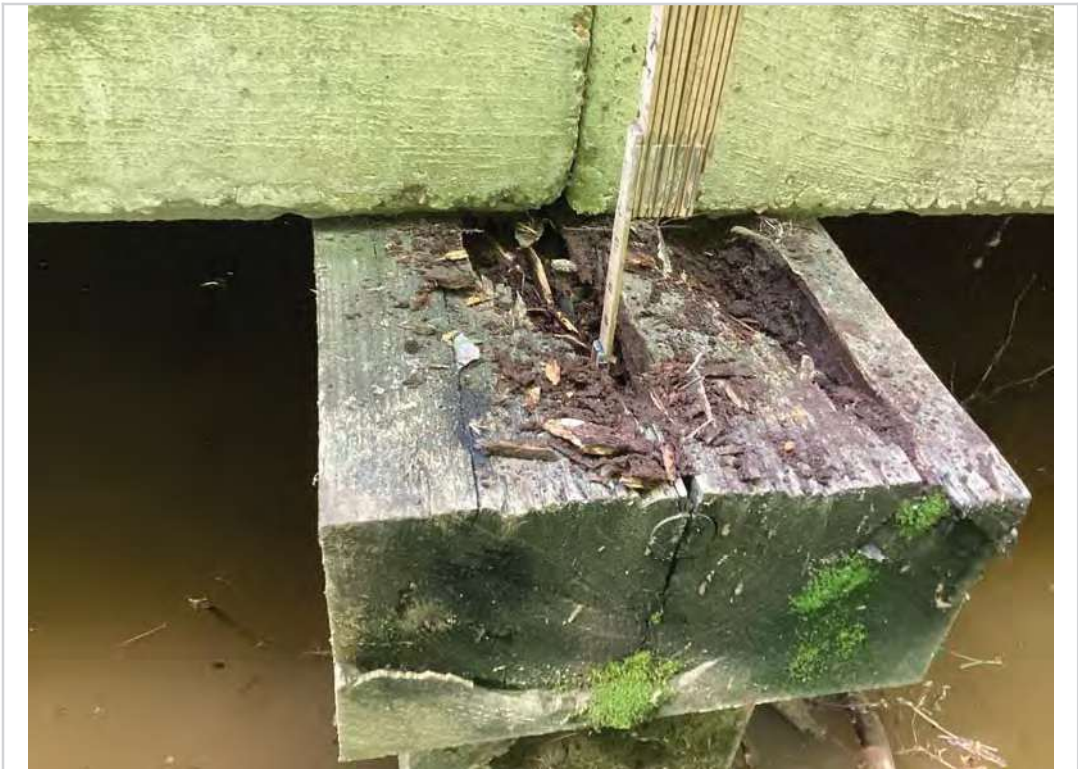
Bent 1 cap "A" right side decay
