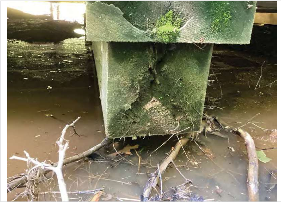
Bent 1 cap "B" right side decay
