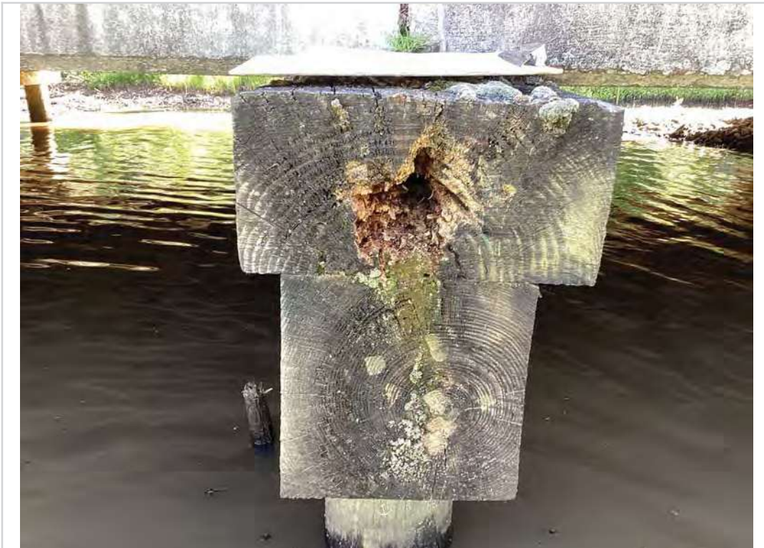
Bent 2 cap A decay on right side
