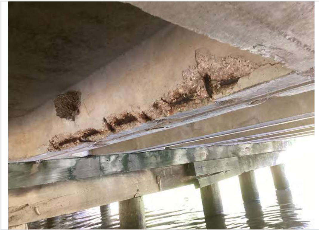
Span #3 PCCS "C" spalling to steel
