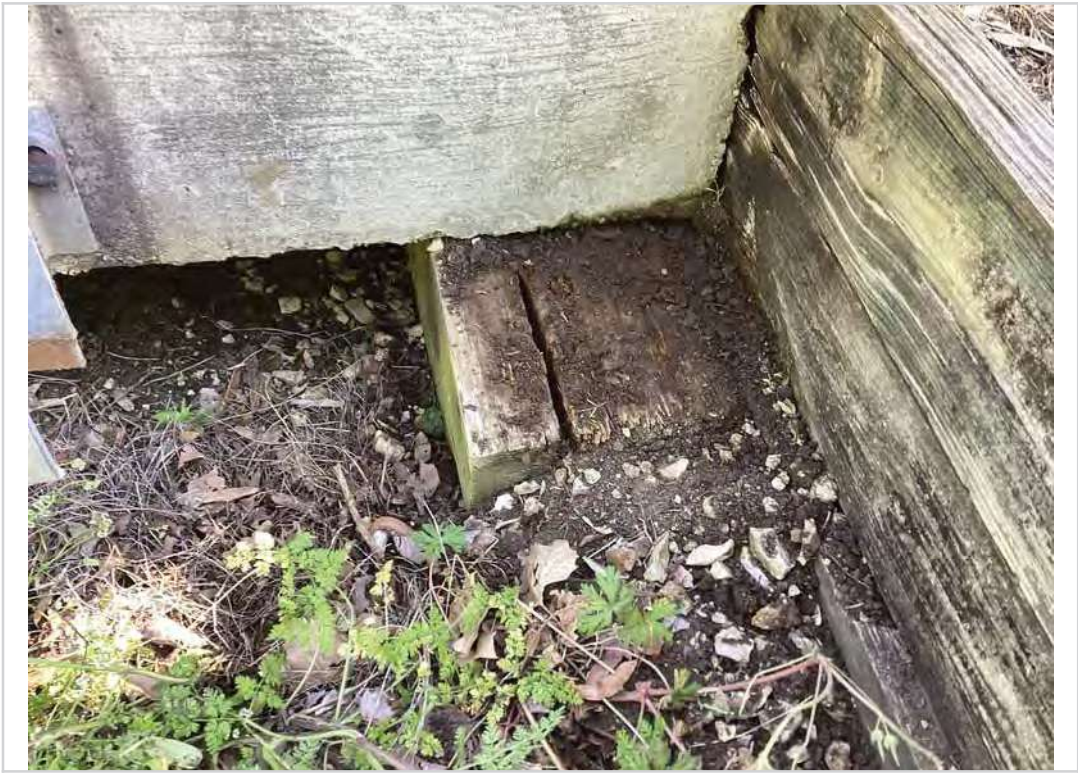
Abutment 1 left side cap decay
