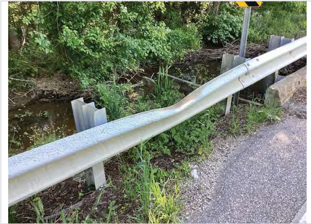
Approach 2 right guardrail
