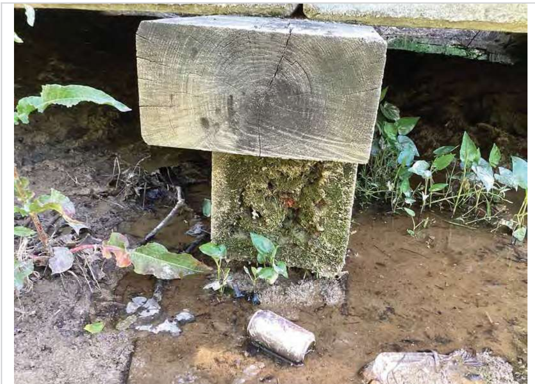
Bent 1 cap "B" left side decay
