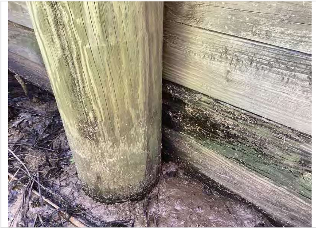
Abutment 2 left wing decay
