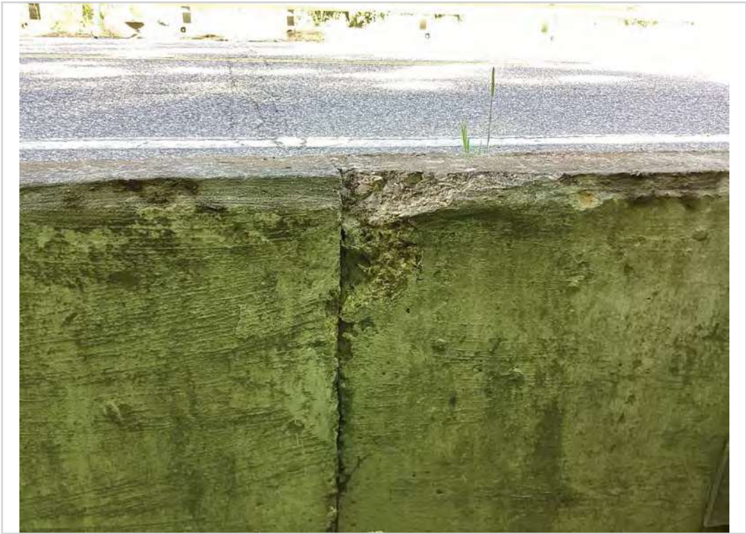
Span 2 right curb spalling
