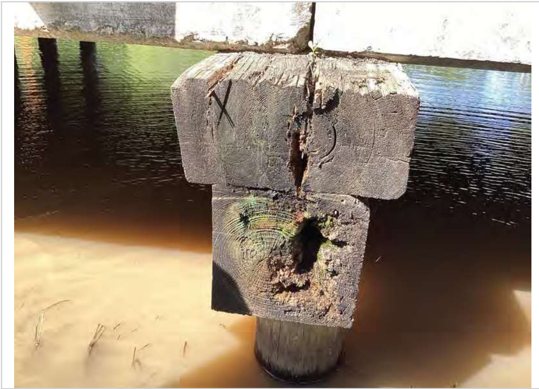
Bent 2 left side decay on cap A & B
