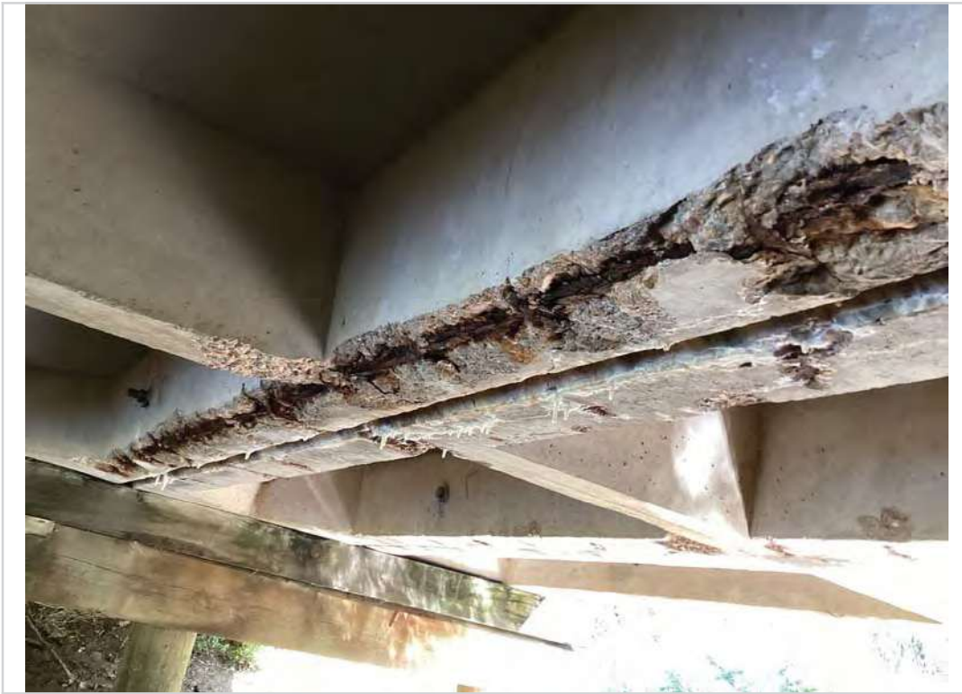
Span 2 slab "C" heavy spall to steel
