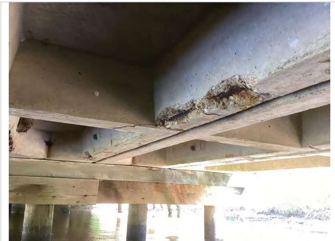
Span #3 PCCS "C" spalling to steel
