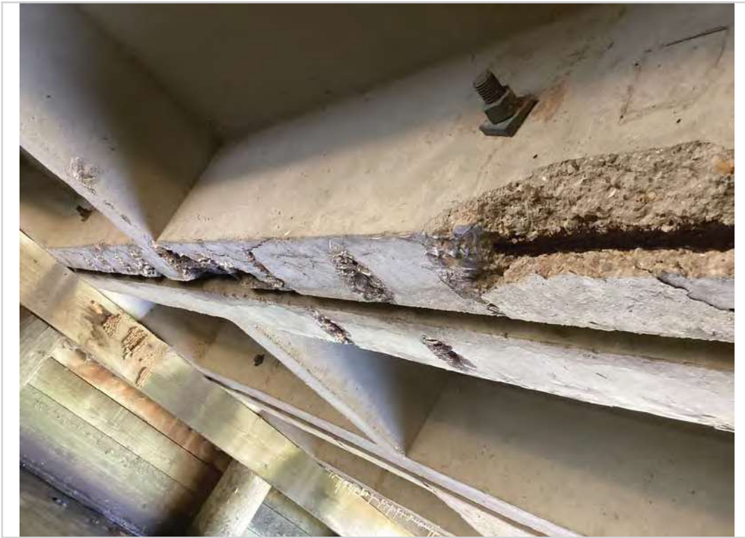
Span #5 PCCS "E" spalling to steel
